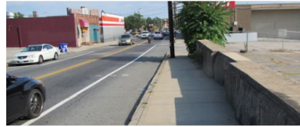
Left: (Before) You can see how stormwater has no-where to go, except into catch basins on the street connected directly to the Woonasquatucket River.
